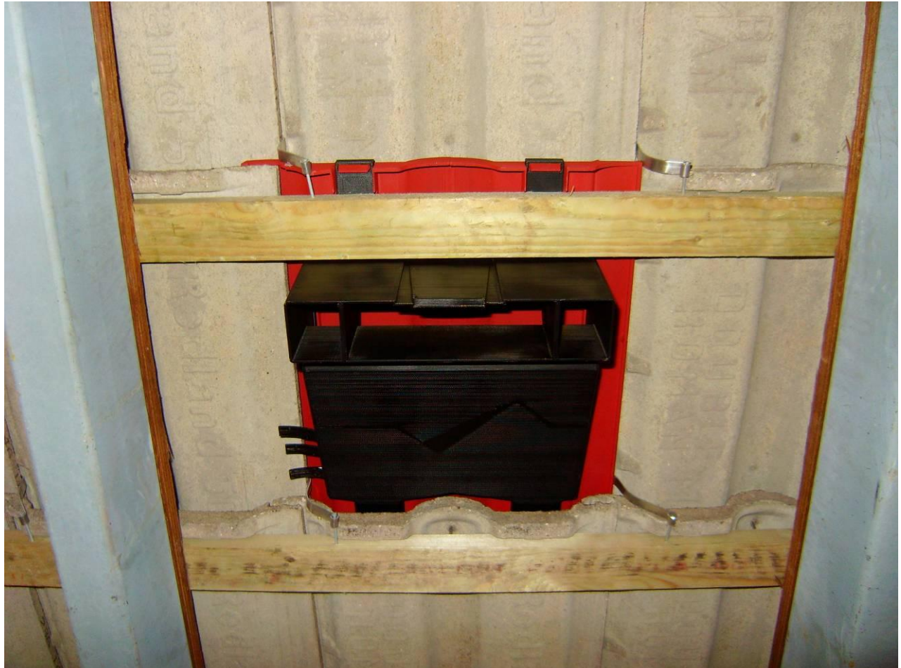
Figure 2 An underside view of the Manthorpe large format concrete interlocking tile vent installed in the test roof
